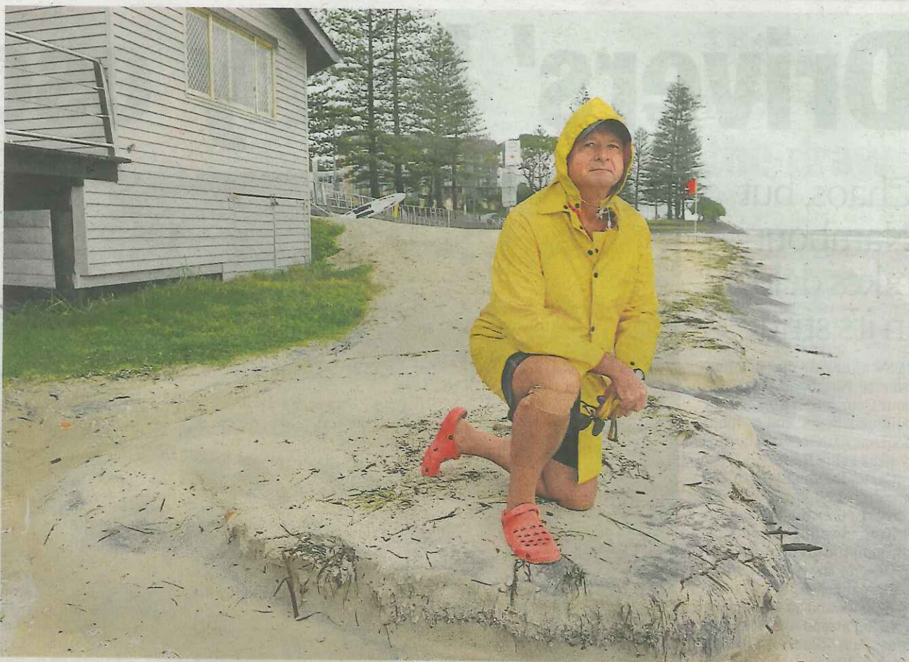
WATCHFUL: Paul Seto, of Ithaca Caloundra Life Saving Club House, inspects erosion at rear of the clubhouse.
